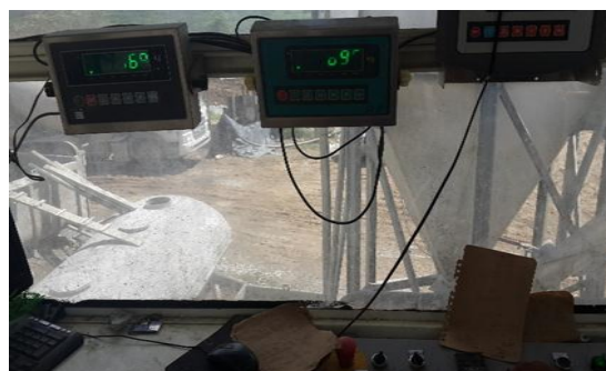
Figura 8. Panel de Control
