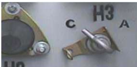
Figura 20 Seccionador Pad Mounted.
