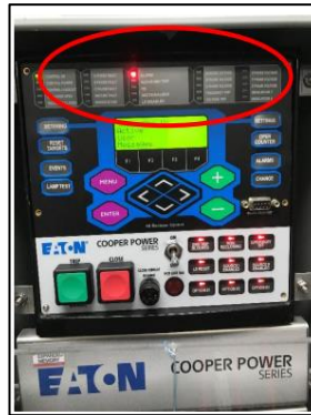
Figura 2. 11. Control Form 6 Recloser Fuente. (EATON Powering Business Worldwide, 2020)
