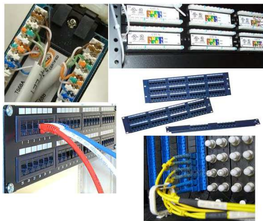
Figura 2.35: Bastidores o Patch Panel
