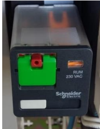
Figura No. 40 Breaker de control
