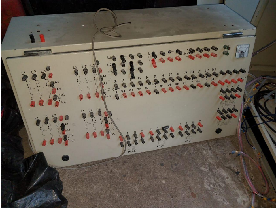
Figura 38. Panel de control- Caja de control
